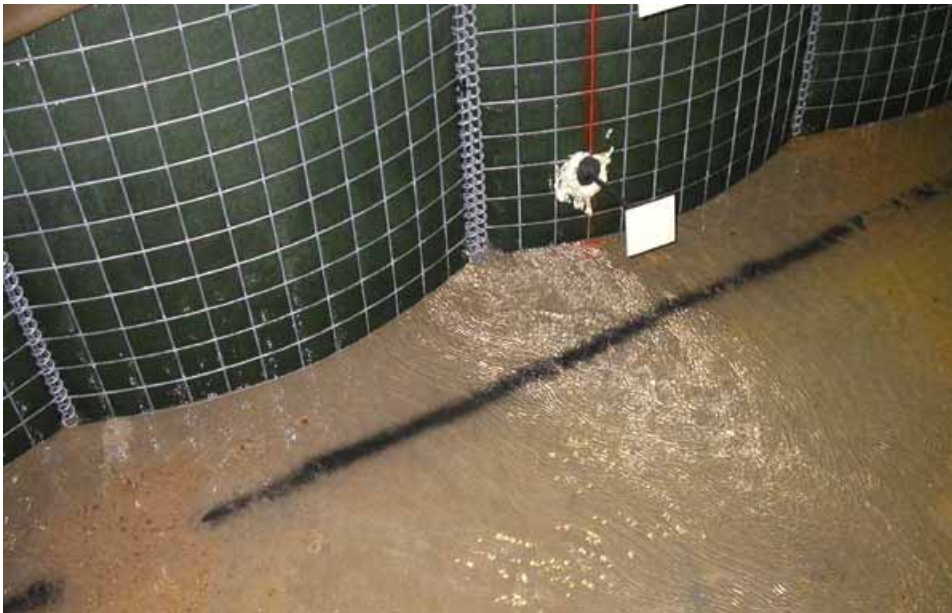
Figure 2-77. Seepage at vertical joint and wall base
