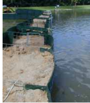
Figure 3-87. 11 June 2004, 4.0 ft of water against structure
