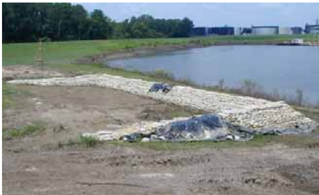
Figure 3-57. Structure after being submerged
