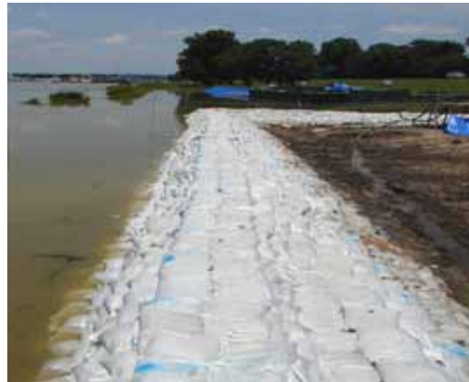
Figure 3-46. 5 June 2004, 2.3 ft of water against structure
