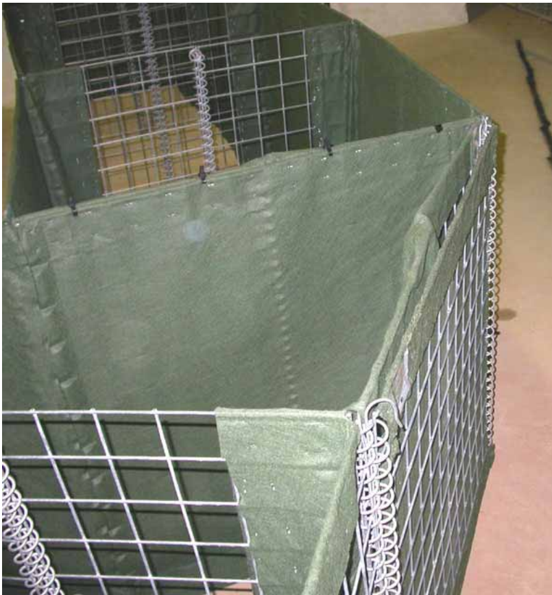
Figure 2-49. Top view of angled unit at intersection of left and center walls
