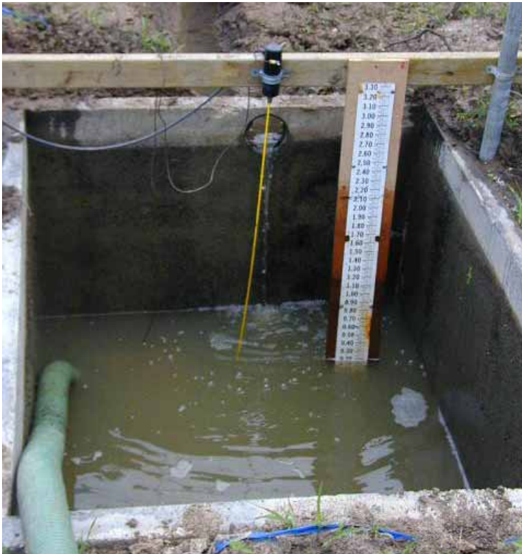
Figure 3-11. Concrete sump with fixed-mount staff gage and capacitance water level sensor
