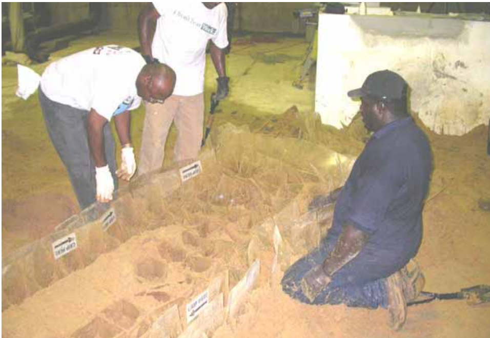
Figure 2-179. Preparing to remove one of second layer grid units. Note bandaged wrists to prevent cuts and scrapes from grid units
