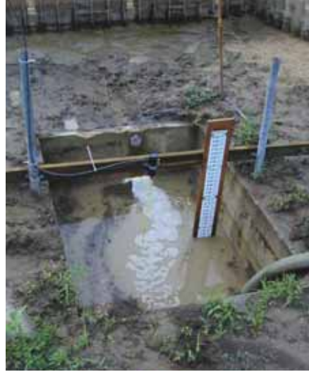
Figure 3-121. Seepage collection in sump tank
