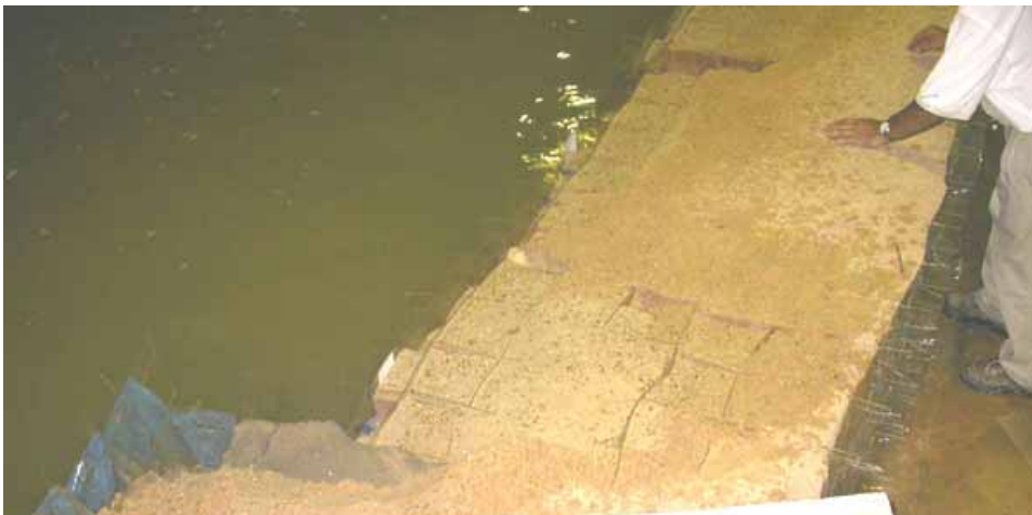
Figure 2-143. Surface erosion from wave action
