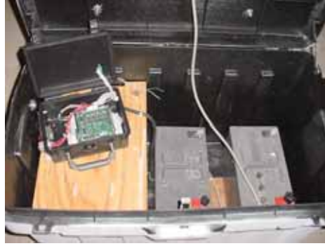
b. Battery power supply
