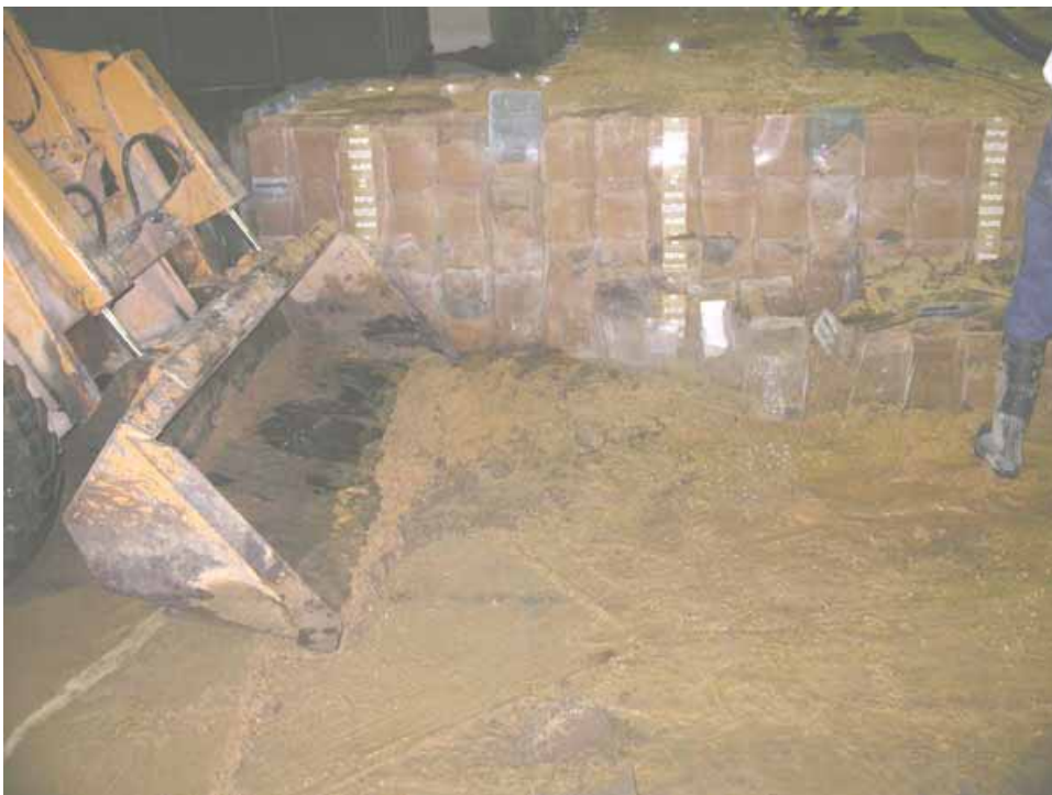
Figure 2-162. Scooping up eroded sand along toe grid units
