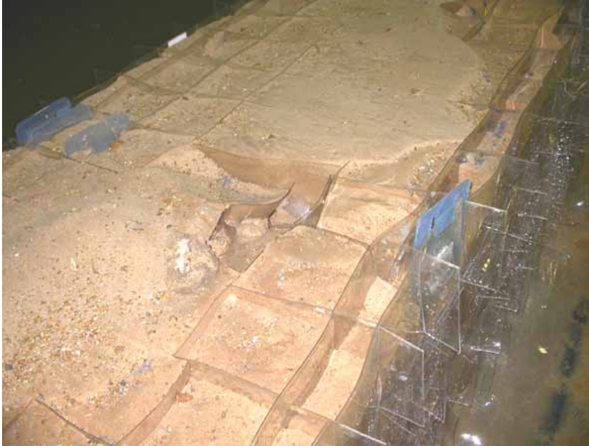
Figure 2-150. Close-up of surface erosion on left wall
