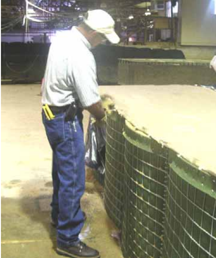
Figure 2-89. Cutting cable ties and removing top cover
