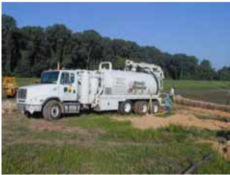
Figure 3-135. Rented vacuum truck
