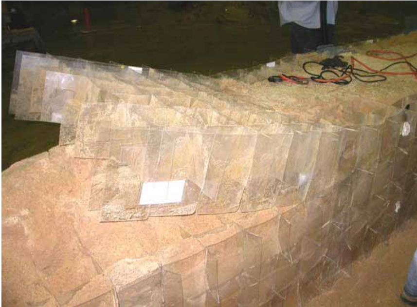
Figure 2-173. Loosened grid unit
