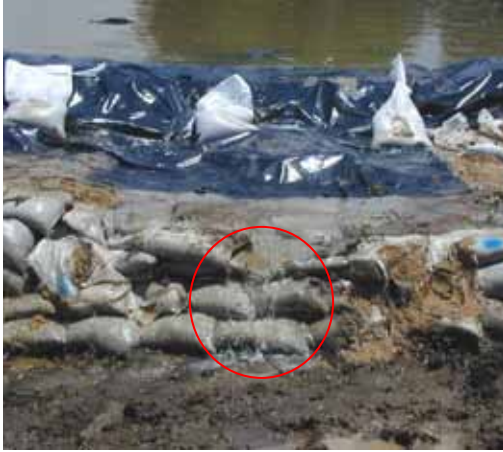
Figure 3-49. 7 June 2004, seepage through structure
