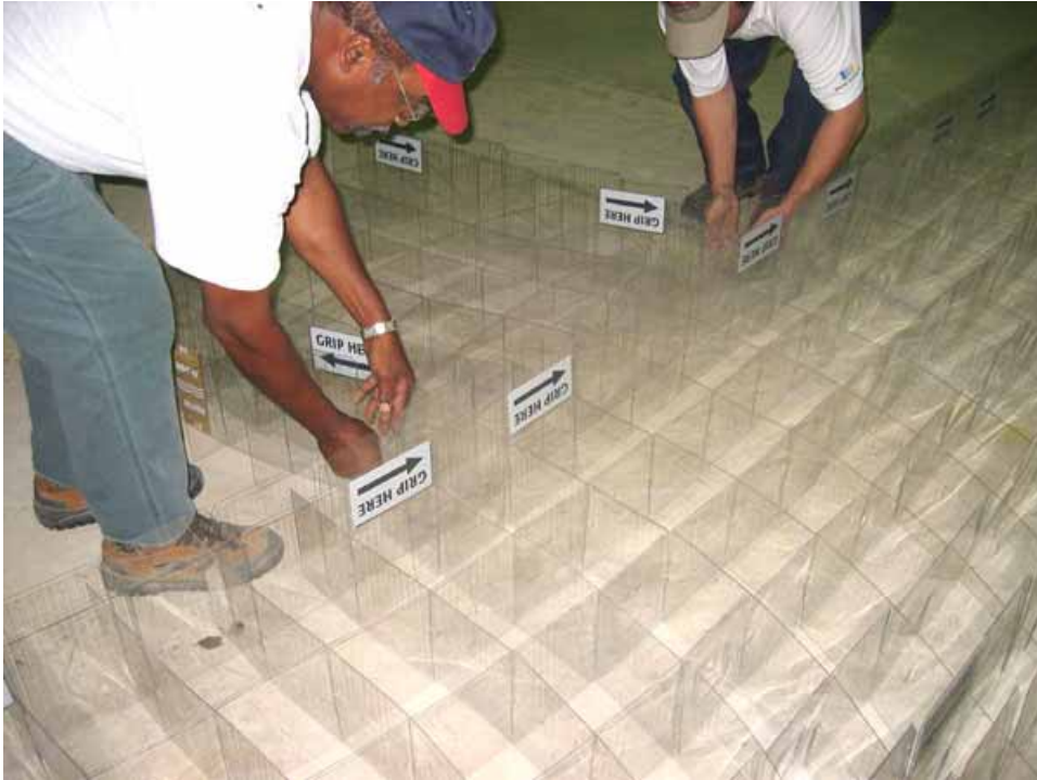
Figure 2-107. Connecting right wall to center wall grid cells, viewed from pool side
