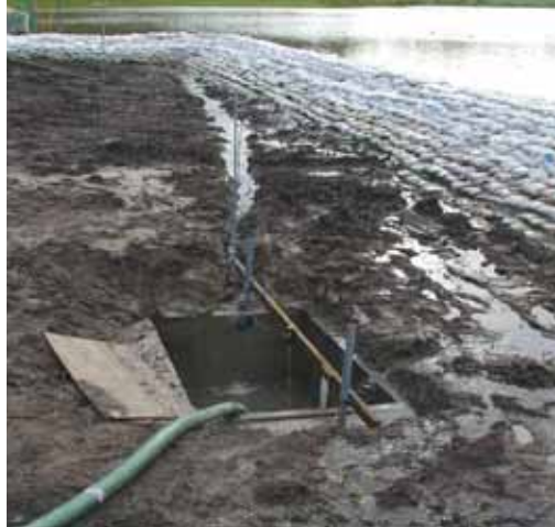
Figure 3-53. Seepage on protected side
