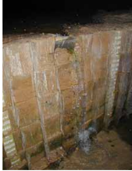
Figure 3-129. Overtopping of RDFW structure
