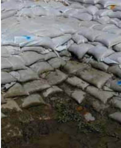
Figure 3-52. Seepage through structure
