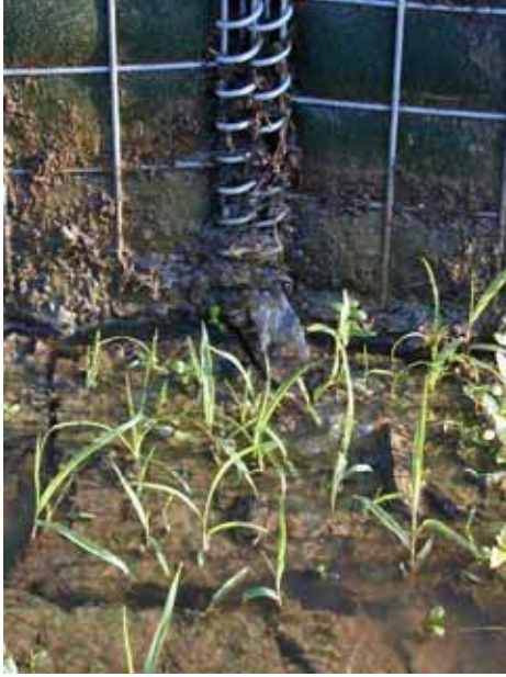
Figure 3-89. Seepage through joints
