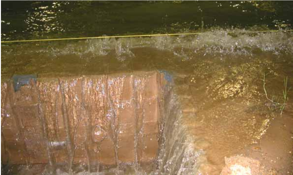
Figure 2-148. Sporadic wave overtopping at intersection of right and center walls
