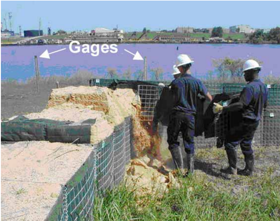
Figure 3-12. Staff gages positioned outside structure for visually monitoring water level changes
