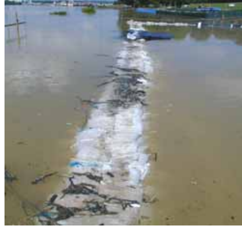
Figure 3-50. 7 June 2004, overtopped structure
