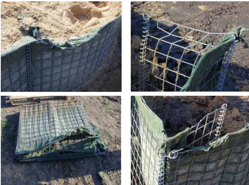
Figure 3-104. Units damaged during removal process
