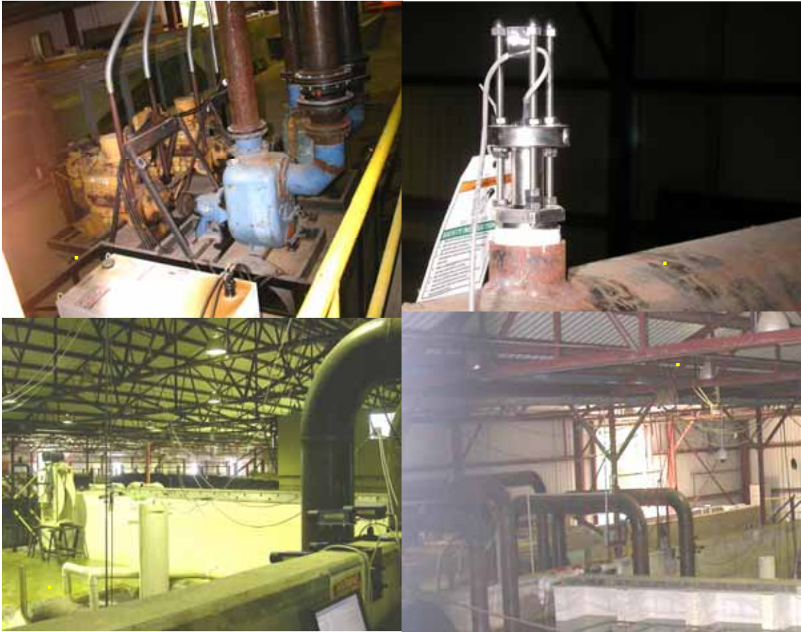
Figure 2-3. Pumping system used for overtopping, 12 in. diam. Top left: diesel pumps. Top right: flow meter. Bottom left: pipes leaving basin to pumps. Bottom right: pipes from basin to pumps and back to basin
