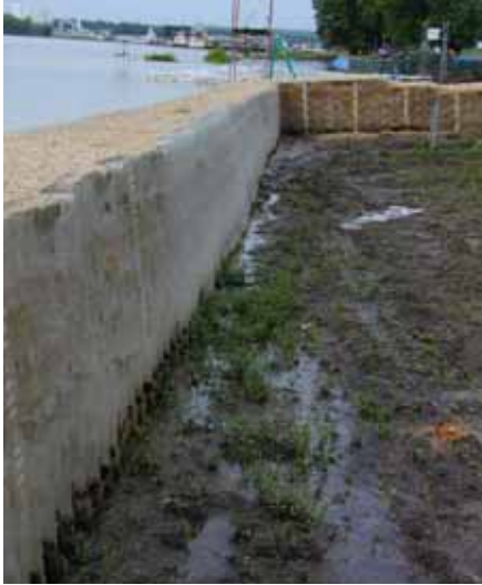
Figure 3-120. Seepage behind RDFW structure
