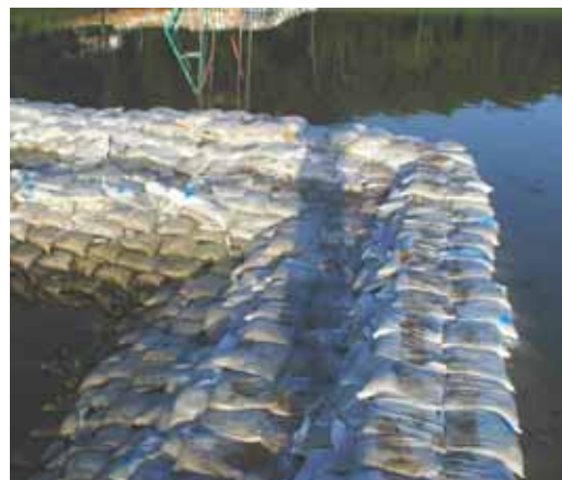
Figure 3-48. 7 June 2004, structure overtopping
