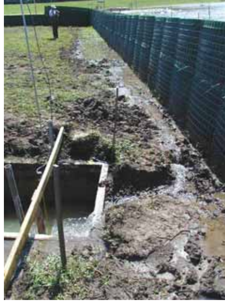
Figure 3-90. Seepage on protected side
