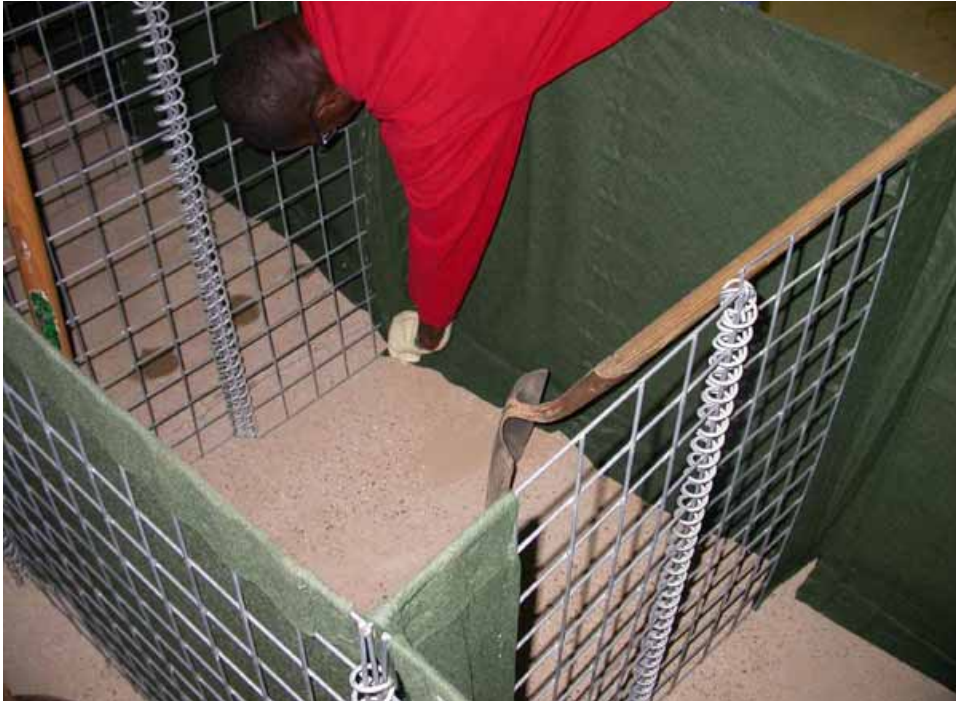
Figure 2-52. Securing flaps against concrete floor. Note center coils which are prefastened at factory
