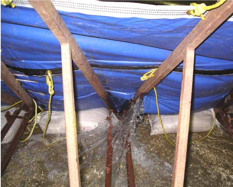
Figure 2-241. Water inflow after large log impact
