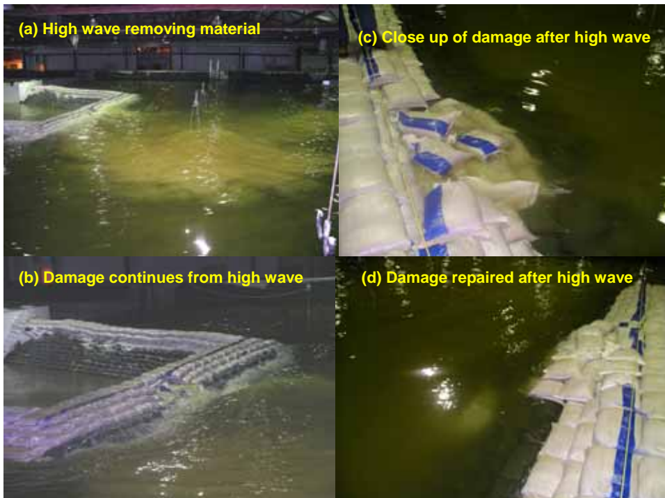
Figure 2-41. Sandbag levee damage and levee after field repair 1
