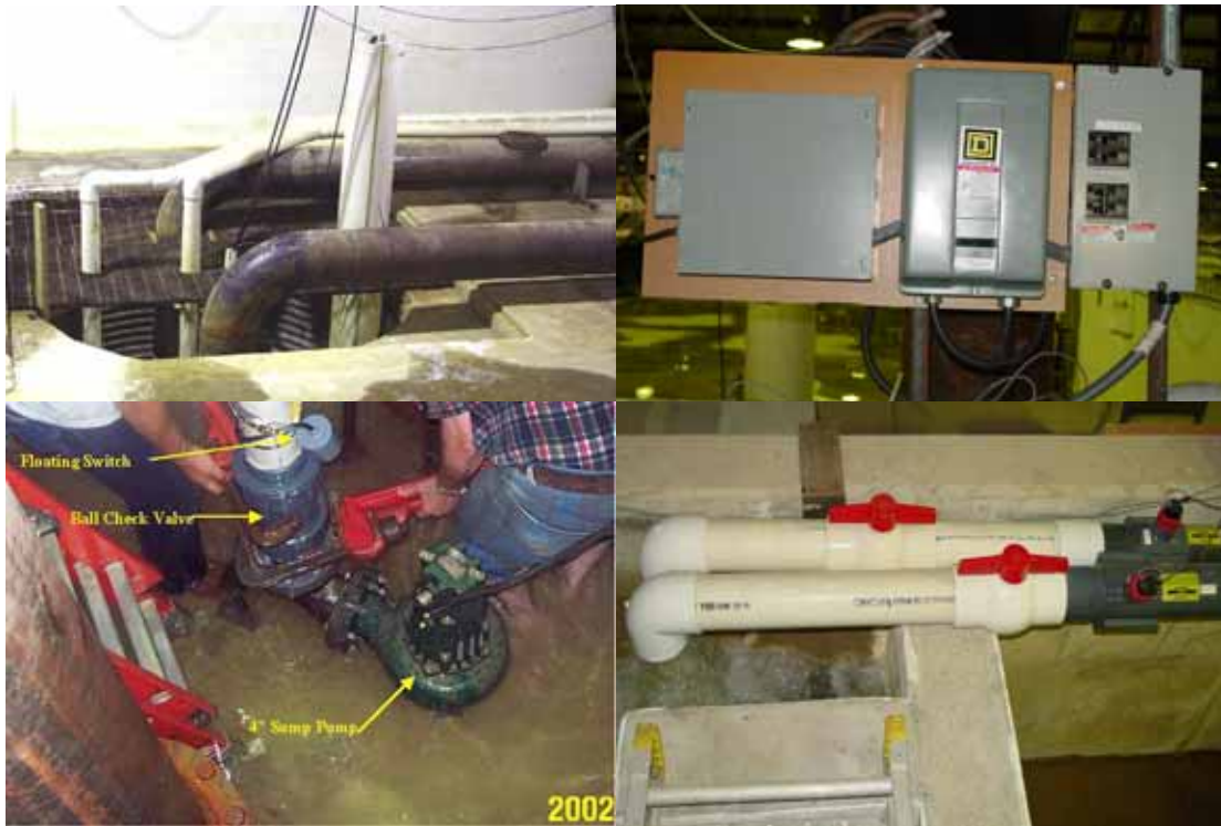
Figure 2-2. Sump pit containing two 4-in. pumps. Top left: top of sump pit. Top right: power control panel. Bottom left: 4-in. pumps in pit. Bottom right: 4-in. valves and flow meters
