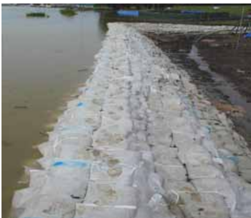
Figure 3-47. 6 June 2004, 3.3 ft of water against structure
